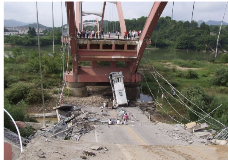
Wuyishan Gongguan Bridge, Fujian (2011) Bridge collapsed after only 12 years of service
