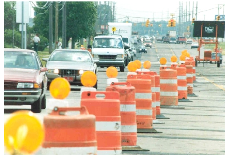
About 40% of Life Cycle Energy for Bridges is Related to Repeated Deck Repairs
